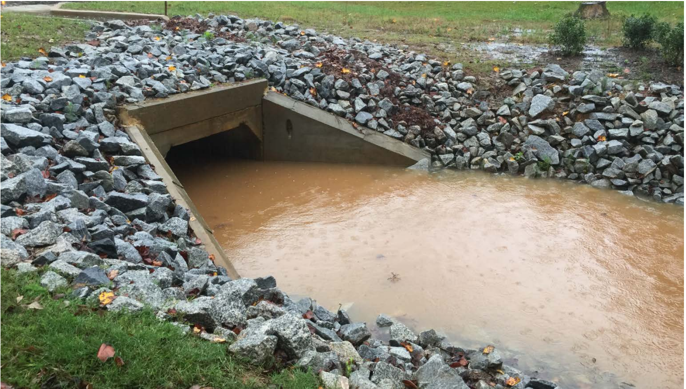
Photo 1: View of outlet side of new culvert. Rain event shows the culvert operating successfully.
