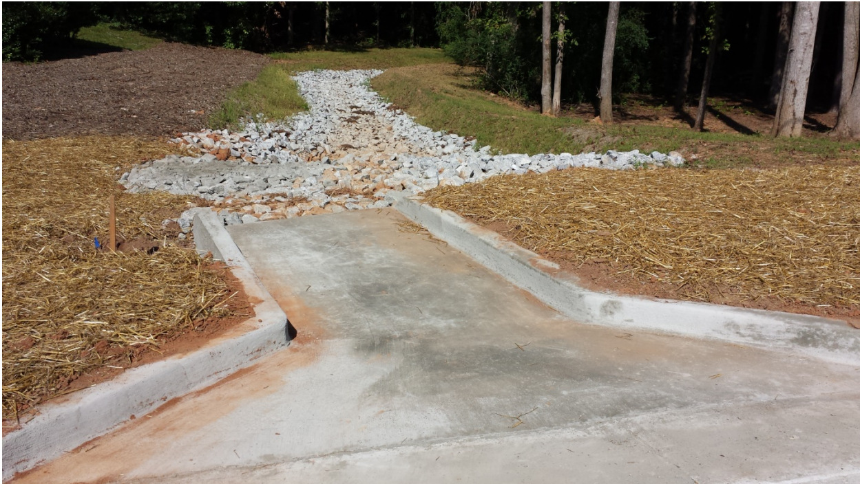
Photo 1: New curb and gutter directs stormwater to flow over new culvert and into the stream. (08/27/2014)
