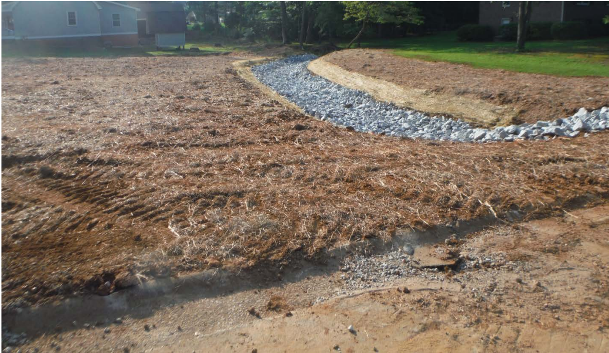
Photo 1: Grading work is underway. Rocks were placed for new stream bed. Materials were placed to help with erosion and sediment control. (06/20/2014)
