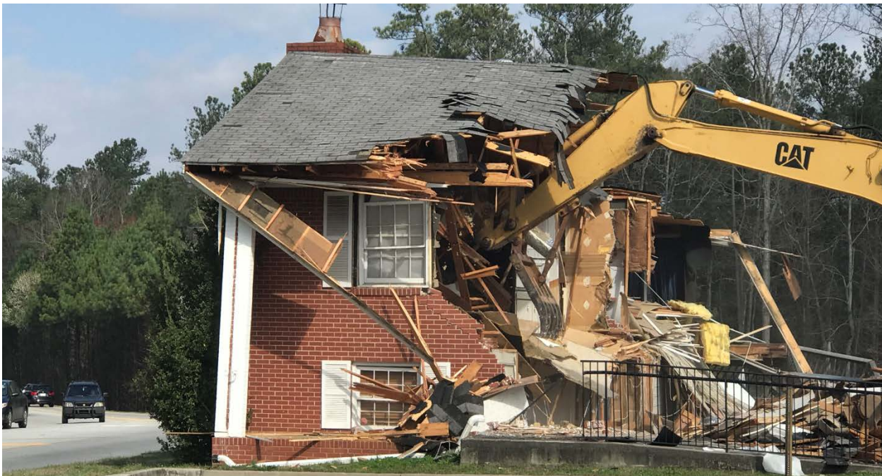
Photo 2: Demolition of the former Department of Driver Services in progress. Future site location of the relocation of Fire Station 4.
