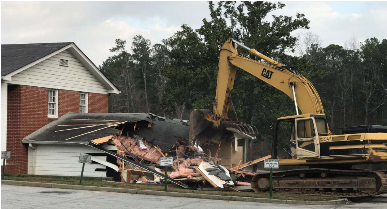
Photo 1: Demolition of the former Department of Driver Services in progress. Future site location of the relocation of Fire Station 4.
