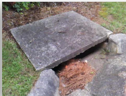
Inaccessible Catch Basin Lid
