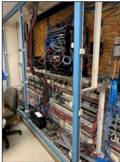
Figure 9. Existing control network wiring at Crosstown WTP Plant Operator Room
