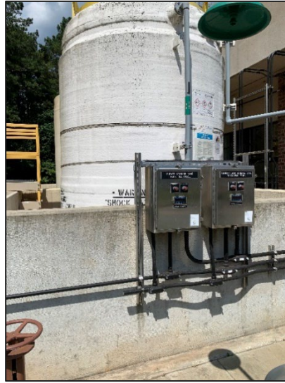
Figure 10. Outdoor Chemical Tanks at Crosstown WTP
