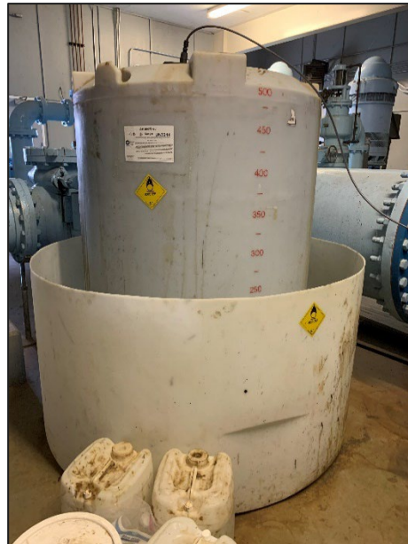
Figure 11. Permanganate Tank at Lake Horton Raw Water Pump Station
