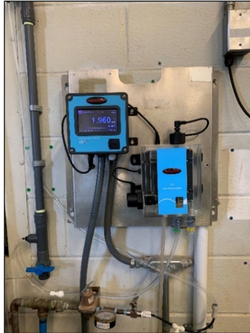
Figure 2. Monitoring Instrument at South Fayette WTP Finished Water Pump Station
