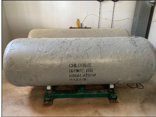
Figure 7. Chlorine Cylinders at South Fayette WTP Chlorine Room
