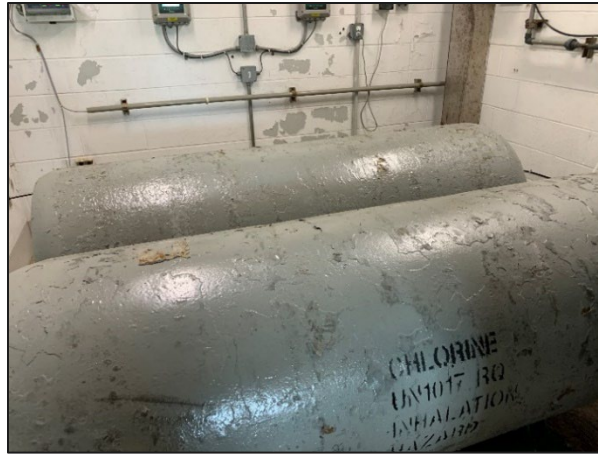
Figure 8. Chlorine Cylinders at Crosstown WTP Chlorine Room
