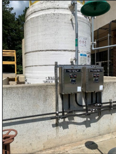
Figure 4. Outdoor Chemical Tanks at Crosstown WTP
