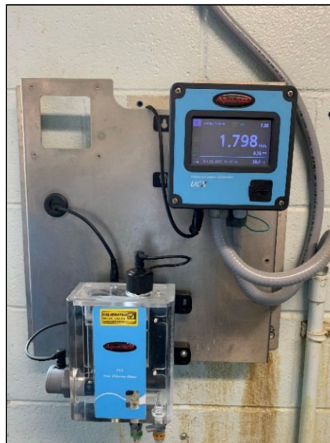
Figure 3. Monitoring Instrument at Crosstown WTP Finished Water Pump Station
