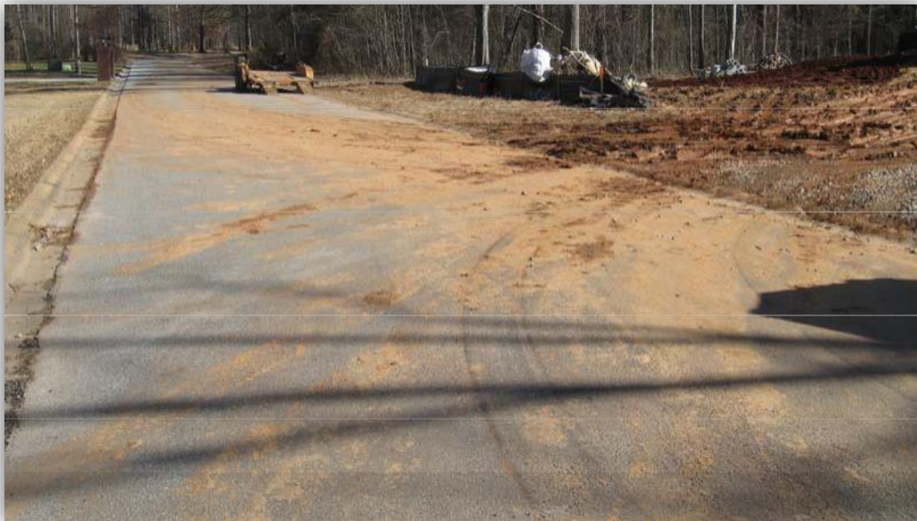
(Mud in the road can cause so many issues)
