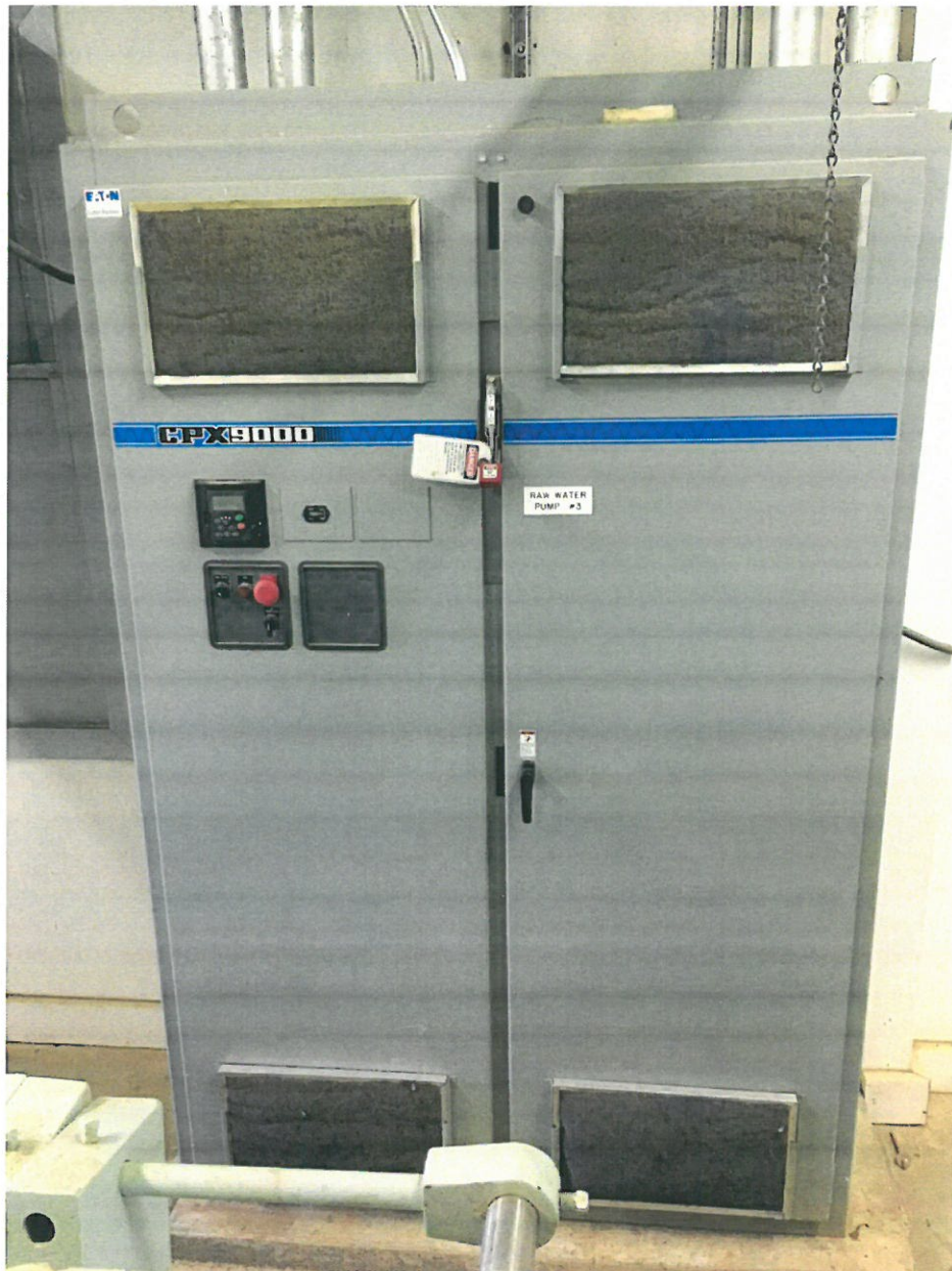
Figure 5 Flint River Pump 3 Drive Cabinet Exterior
