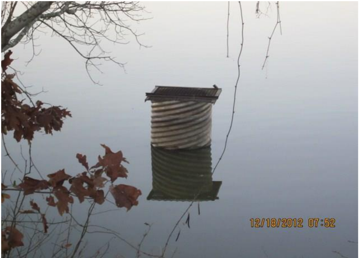
2012 PHOTO: VIEW OF ORIGINAL CORRUGATED METAL OVERFLOW PIPE. LAKE LEVEL IS ABOUT 2 FEET BELOW NORMAL POOL DUE TO LEAKAGE THROUGH THE PIPE.
