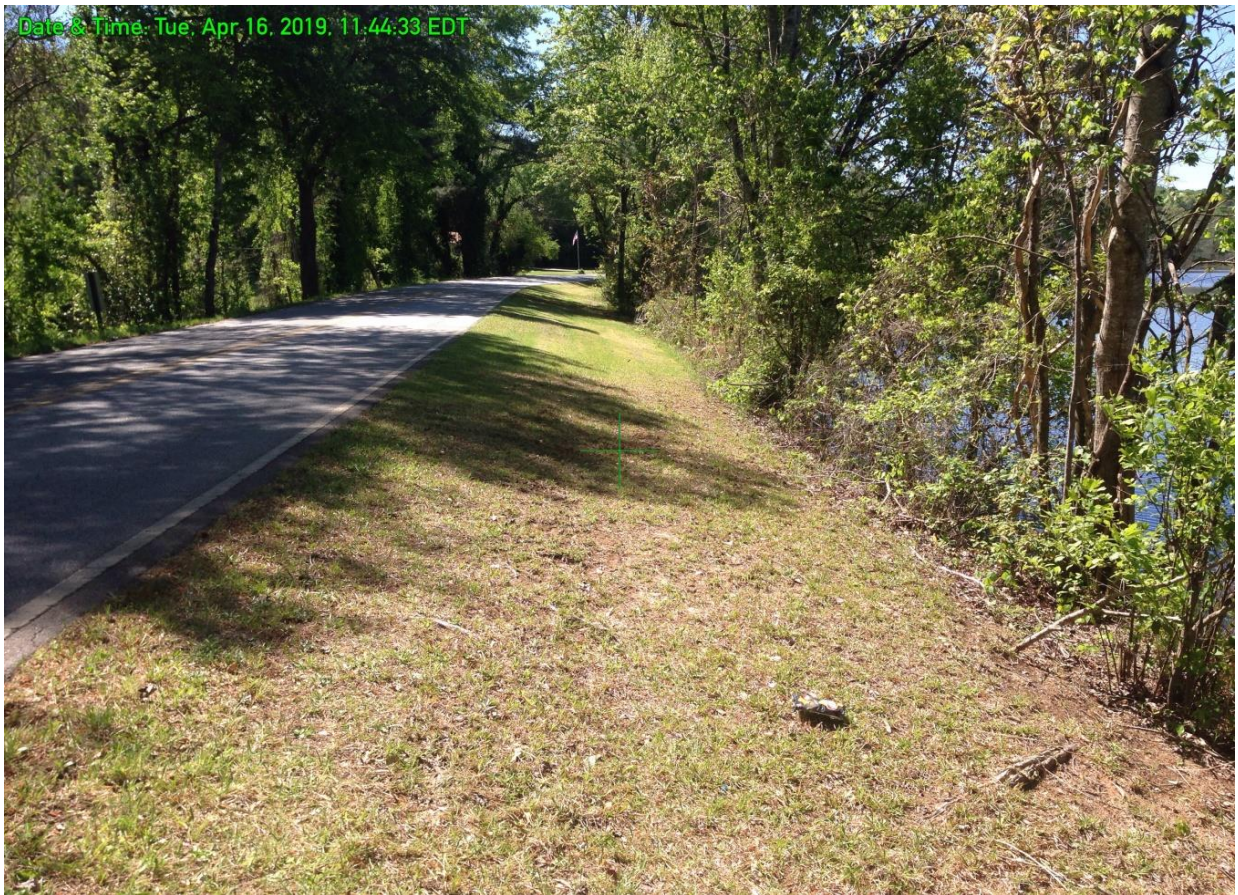
VIEW LOOKING SOUTH ALONG THE UPSTREAM SLOPE FROM NEAR THE NORTH END OF THE DAM.
