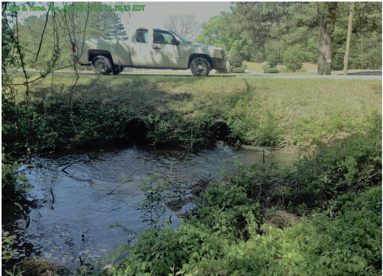
VIEW OF TWO CONCRETE PIPES LOCATED NEAR THE NORTH (LEFT) END OF THE DAM. PIPES ARE CURRENTLY SERVING AS SERVICE SPILLWAY (ORIGINALLY EMERGENCY SPILLWAY PIPES).
