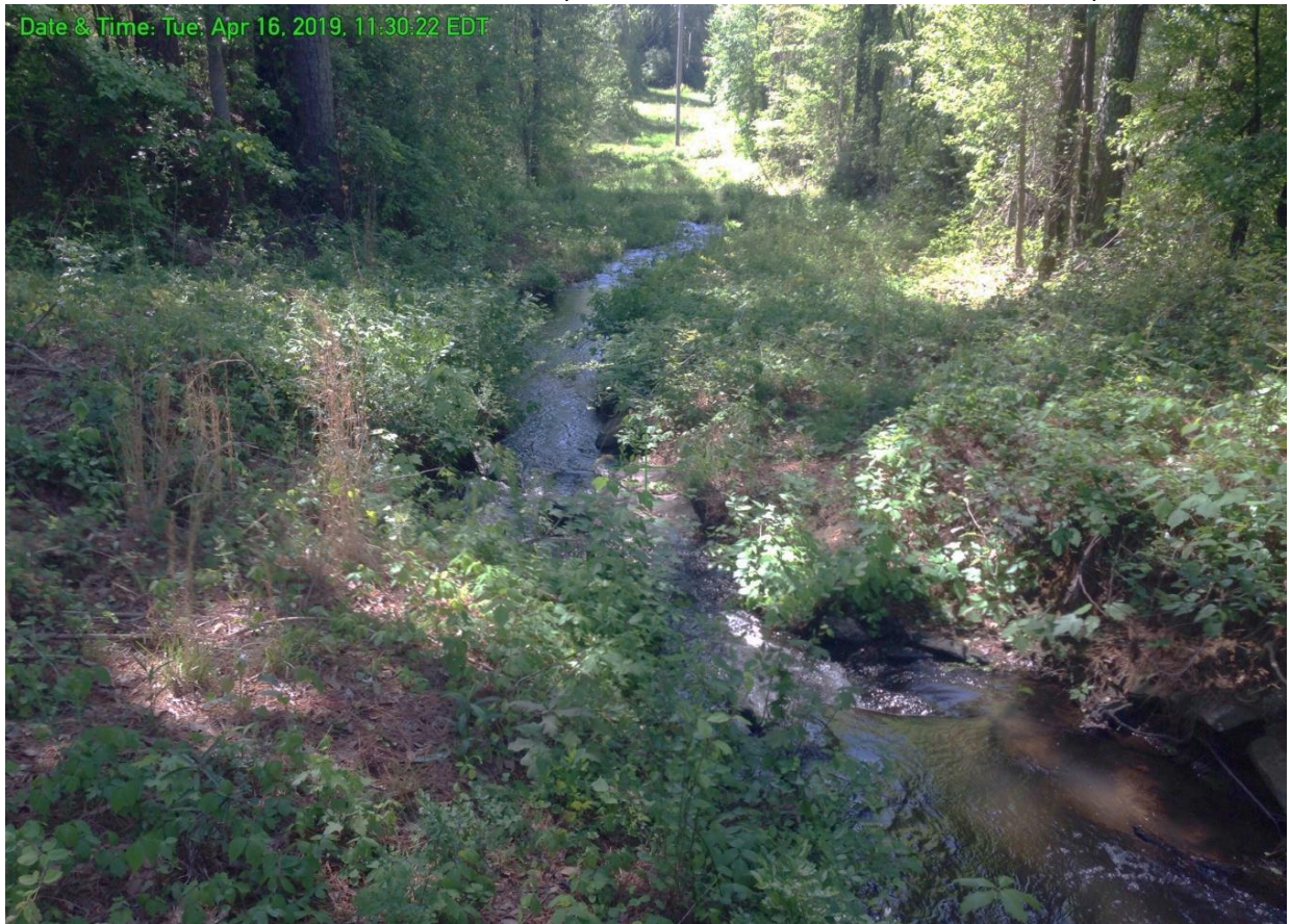
VIEW FACING SOUTH ALONG THE DOWNSTREAM TOE OF DAM WITHIN POWERLINE EASEMENT. WATER FLOWS WITHIN THE EASEMENT FOR ABOUT 400 FEET BEFORE ENTERING STREAM.
