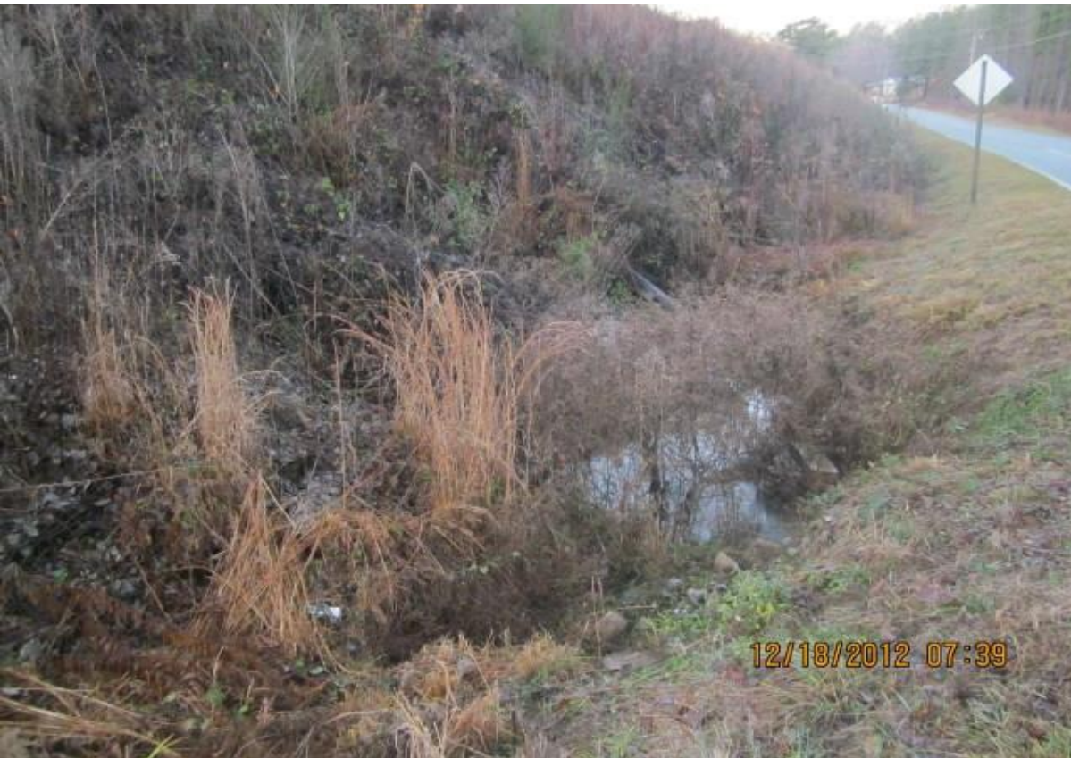
2012 VIEW OF WATER AT THE DOWNSTREAM SIDE OF THE DAM NEAR THE DRAIN PIPE. SIPHON OR PUMP PIPE(S) WERE PRESENT AT THAT TIME. FLOWING WATER OBSERVED ALONG NEELY ROAD.
