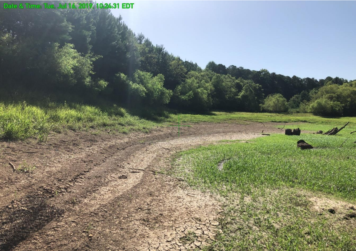
VIEW LOOKING RIGHT ALONG UPSTREAM SHORELINE FROM NEAR LOW LEVEL PIPE WITH LAKE ESSENTIALLY DRAINED.
