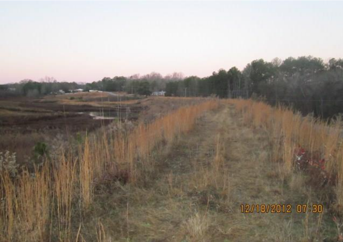
2012 VIEW OF DAM LOOKING RIGHT TO LEFT ALONG THE CREST. VEGETATION WAS BETTER MAINTAINED AT THAT TIME.
