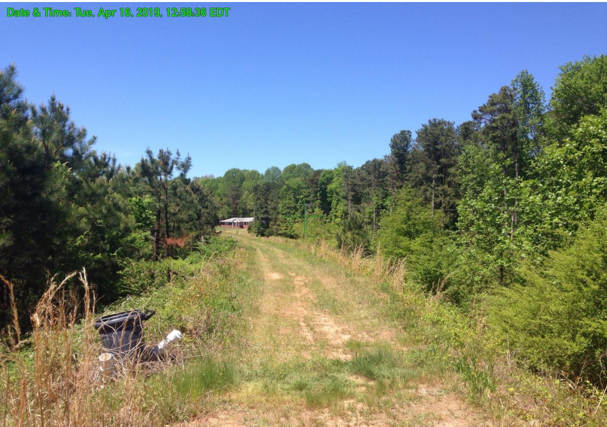
VIEW ALONG THE DAM CREST FROM NEAR THE MID-POINT. REMNANTS OF SIPHONS OR PUMP PIPE PRESENT. RESIDENCE NEAR MIDDLE TOP IS ACROSS NEELY ROAD FROM THE LEFT END OF DAM.
