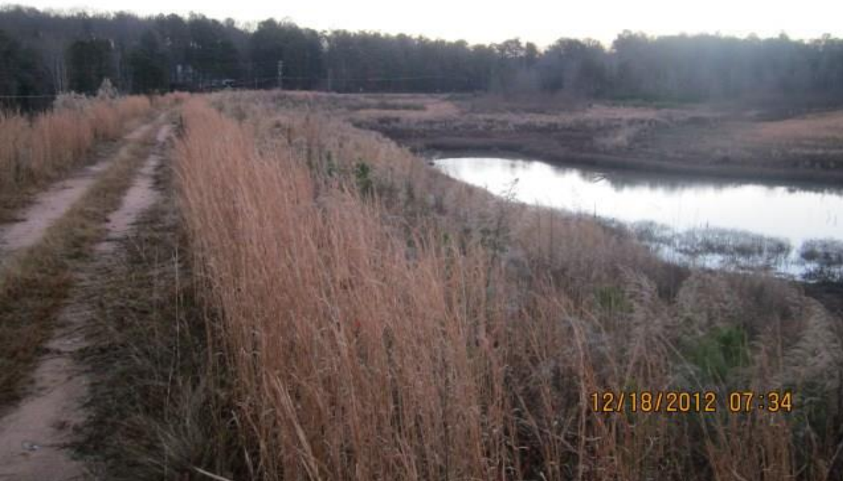
2012 VIEW LOOKING LEFT TO RIGHT ALONG THE UPSTREAM SLOPE AND STANDING POOL.
