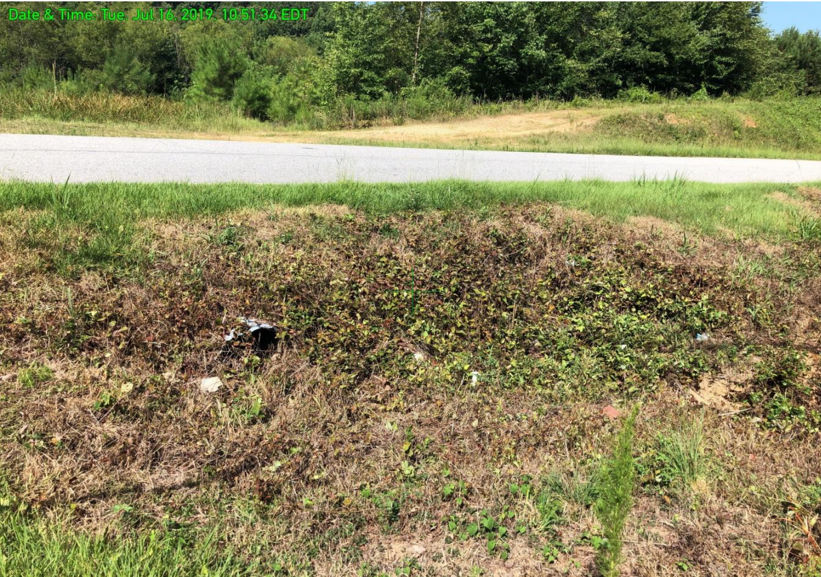
VIEW OF DOWNSTREAM SIDE OF AUXILIARY SPILLWAY PIPE AT NEELY ROAD. THE RIGHT END OF THE DAM CAN BE OBSERVED AT THE TOP OF THE PHOTO ACROSS NEELY ROAD.
