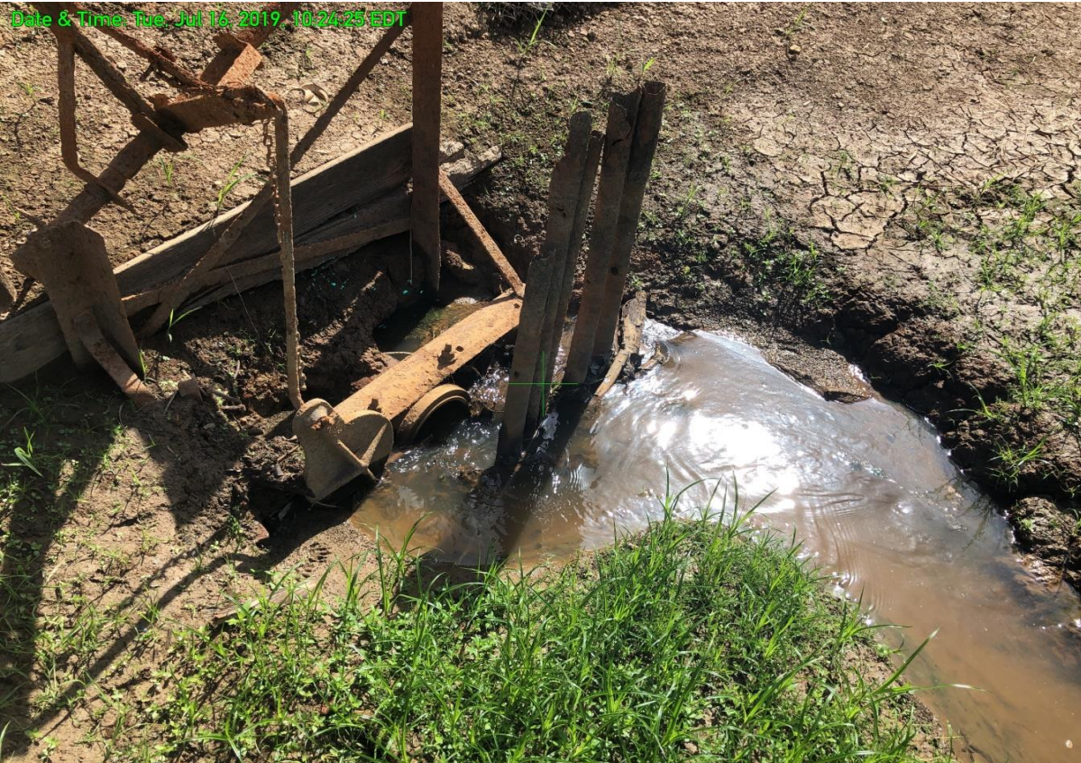
VIEW OF SMALL DIAMETER LOW LEVEL DRAIN PIPE WITH SLIDE GATE OPEN. NORMAL STREAM FLOWS EXIT LAKE AREA THROUGH THIS PIPE. THE OUTLET END OF THIS PIPE WAS NOT LOCATED.
