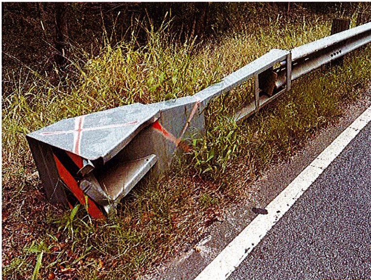
McDonough Road @ Flint River – repair damaged End Treatment
